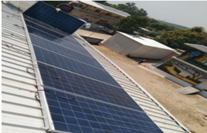
Vena Energy installed a rooftop solar powered system at Earth Saviour NGO, Gurgaon, India
