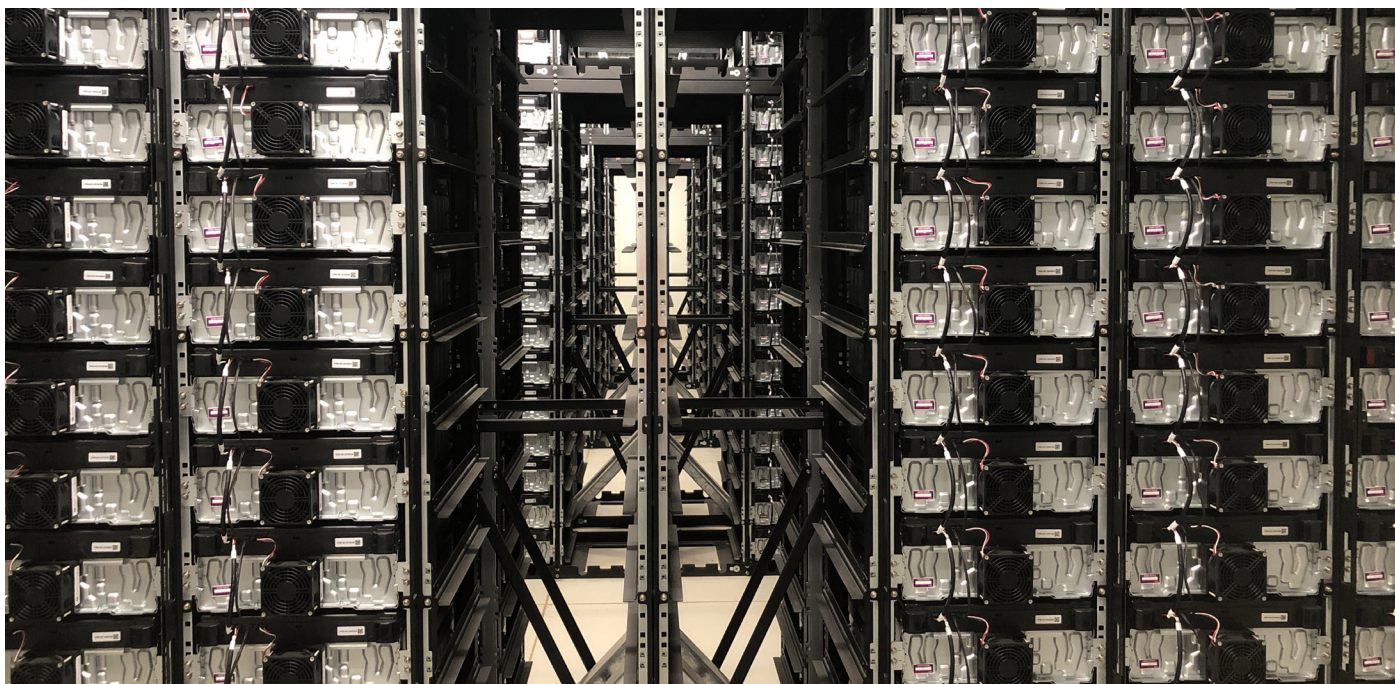
Interior of the Wandoan South Battery Energy Storage System
